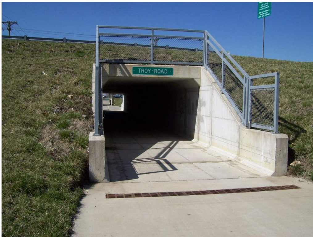
Fig. 3.1 - Example of a culvert underpass on old IL 157 in Edwardsville near the LeClair neighborhood
